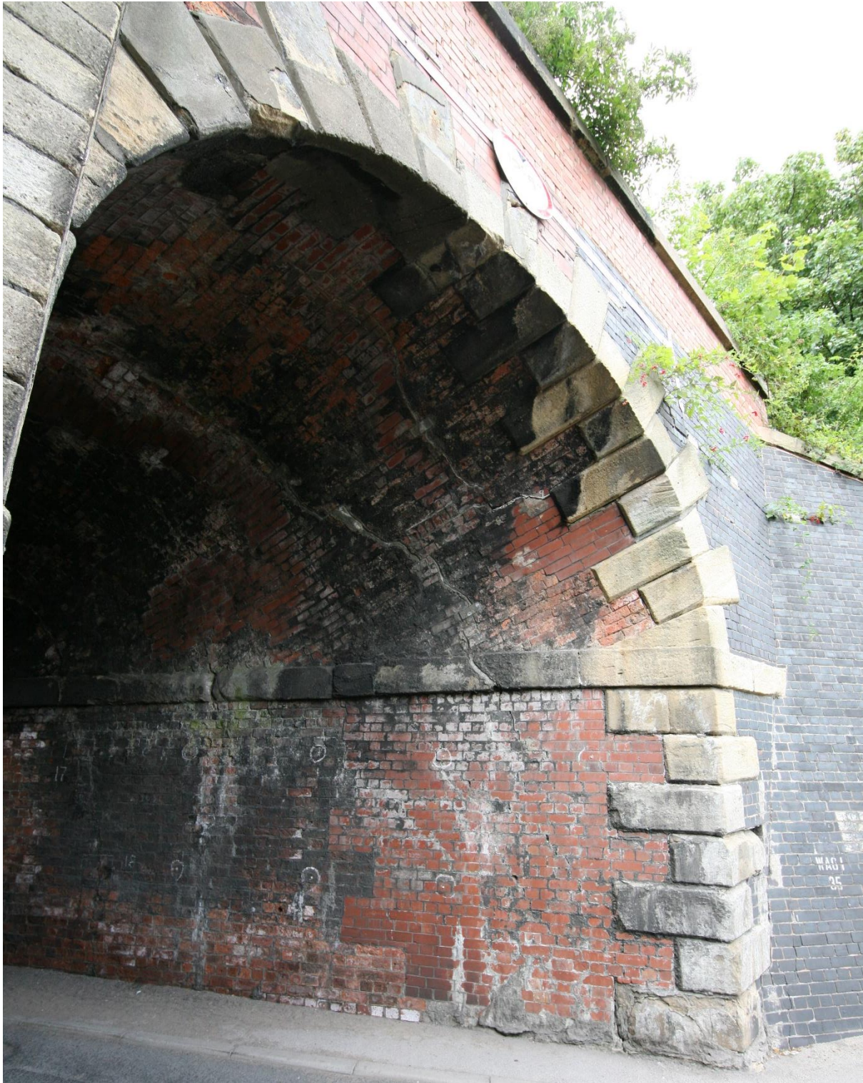
There is red brick patching in both portals. Less here than at the other end below. The cracking is quite a feature though, with cracks right through the stone string course and some step displacement too.
