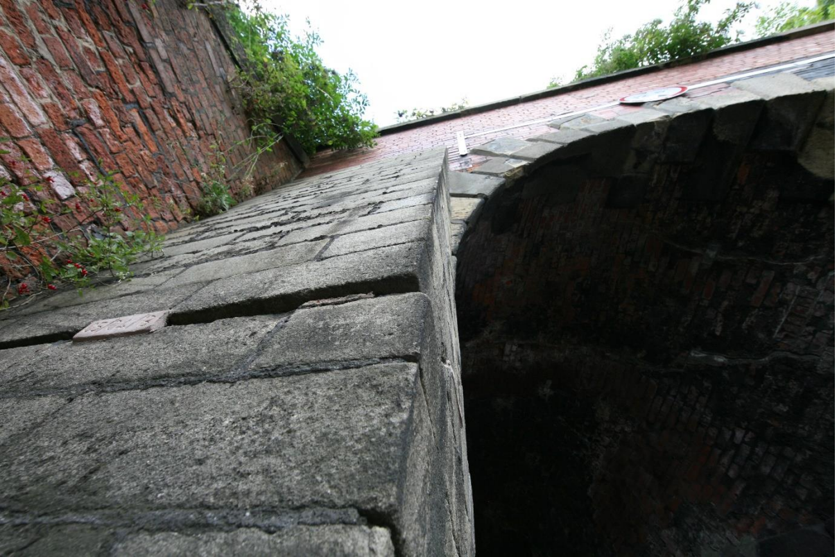
That's quite a joggle in the joint too.
